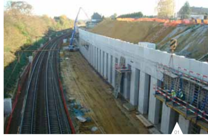
2011 with Franki Foundations producing the first diaphragm walls. This giant site, representing the largest Walloon civil engineering project in recent years, will last for no less than 50 months.
